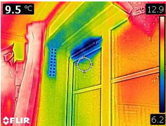
Window trickle vents are a necessary part of the ventilation system. However, the vent in the reveal here, which is adding to heat loss, could potentially be sealed if a better ventilation system was installed - removing wet air from kitchens and bathrooms.
